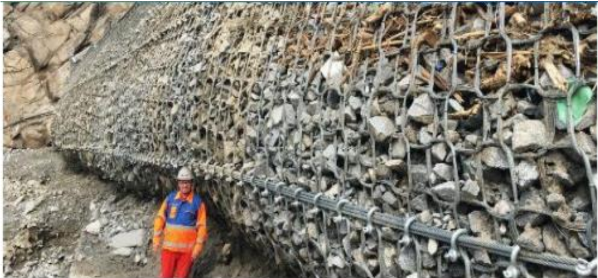
Figure 73: Wire mesh installed to minimise the risk to Skorpion Zinc Mine employees Source: (Tshiningayamwe, 2021)
