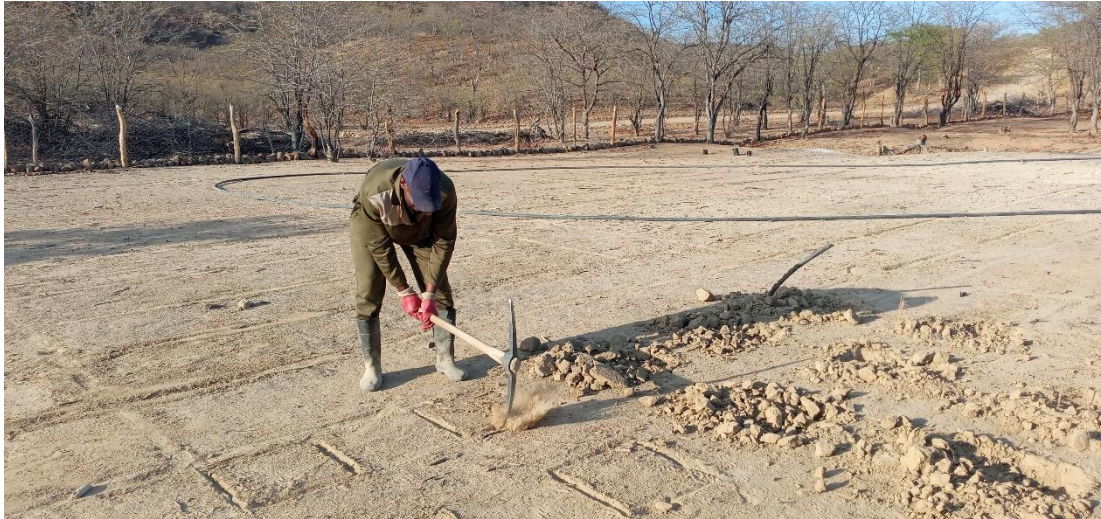
Figure 10. Digging of the seedling holes at 1m apart at the experimental site.
