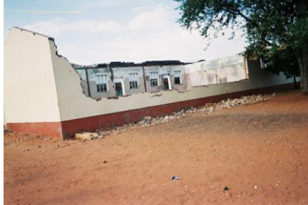
Burnt down classrooms
