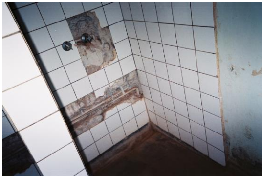
Delay in repairs
