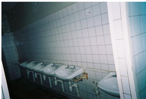
Vandalized and removed sinks and face basins
