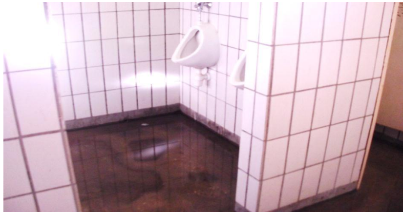
Figure 4.8: Toilet facilities filled with stagnant waters
