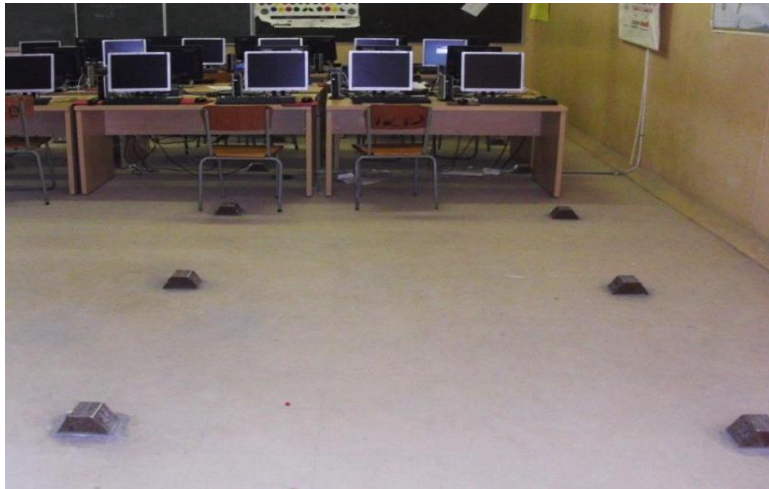
Figure 4.5: The electric sockets on the floor in the computer lab
