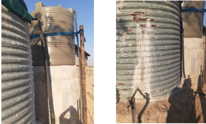
Figure 3.4 & 3.5. Water tanks at Grundorn showing rusting and leaking.
