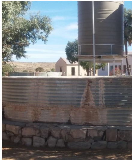
Figure 3.15. The rusted metal sheets around the dam and one of the water tanks at Nico.
