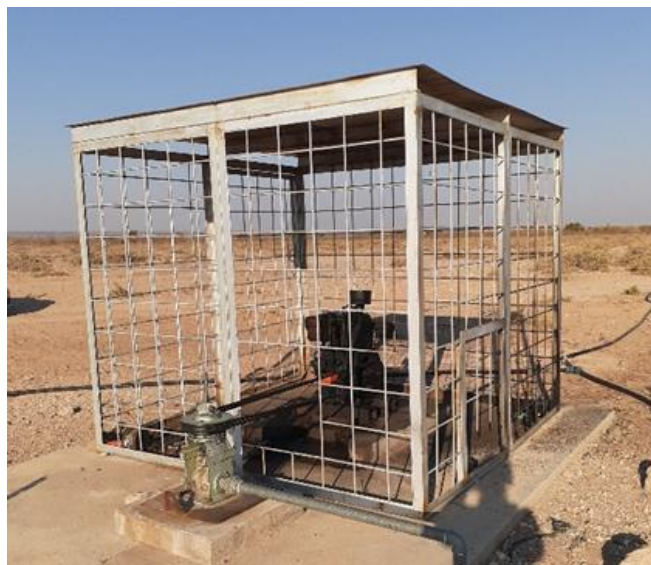
Figure 3.3. Diesel water pump at Grundorn.
