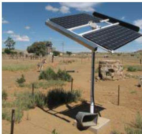
Figure 3.16. Solar powered borehole at Nico.
