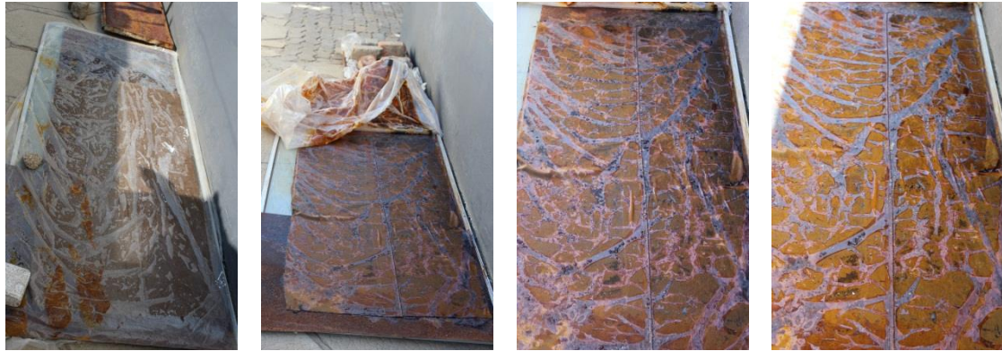
Figure 17 - Rusted panels for trouser. Photographs: By Author
