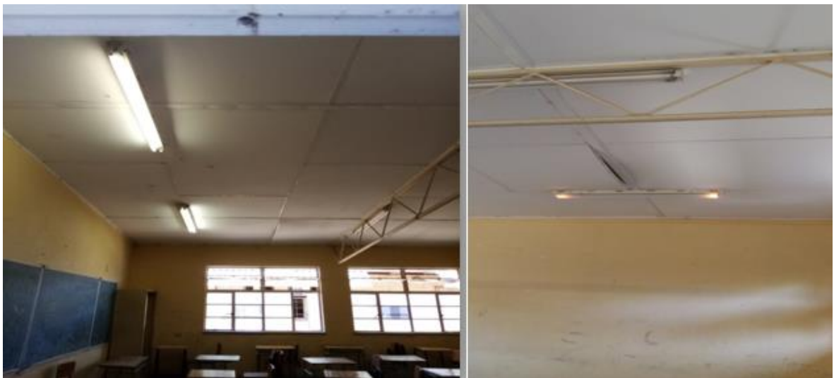
Figure 4.11 Classrooms with Non-working and Flashing Bulbs
