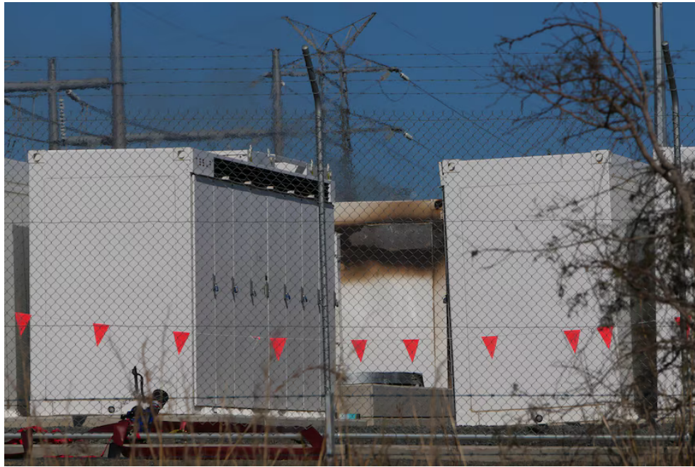
Figure 8. Shows the aftermath of the BESS fire incident in Bouldercombe, Australia [38].
