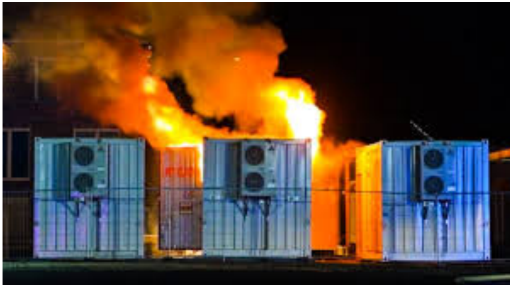
Figure 15. Lithium battery energy storage container caught fire in the business district of Neermoor [46].
