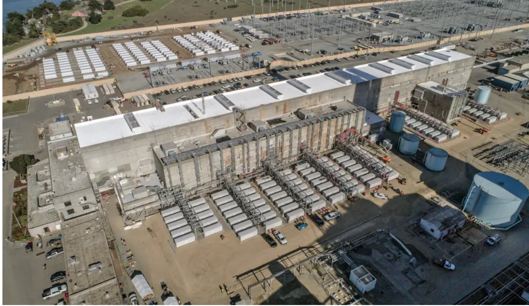
Figure 10. Vistra's Moss Landing energy storage facility (centre) before the incident [41].
