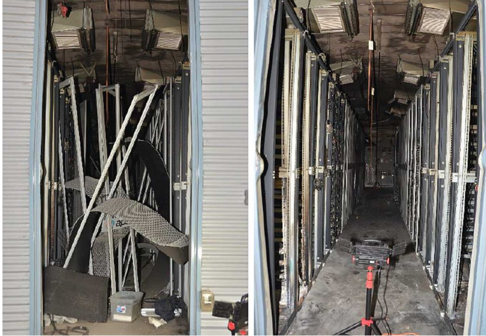
Figure 5. Damage to the BESS’s interior following the explosion (left), and following the removal of debris to allow entry for start of the forensics investigation (right) [37].
