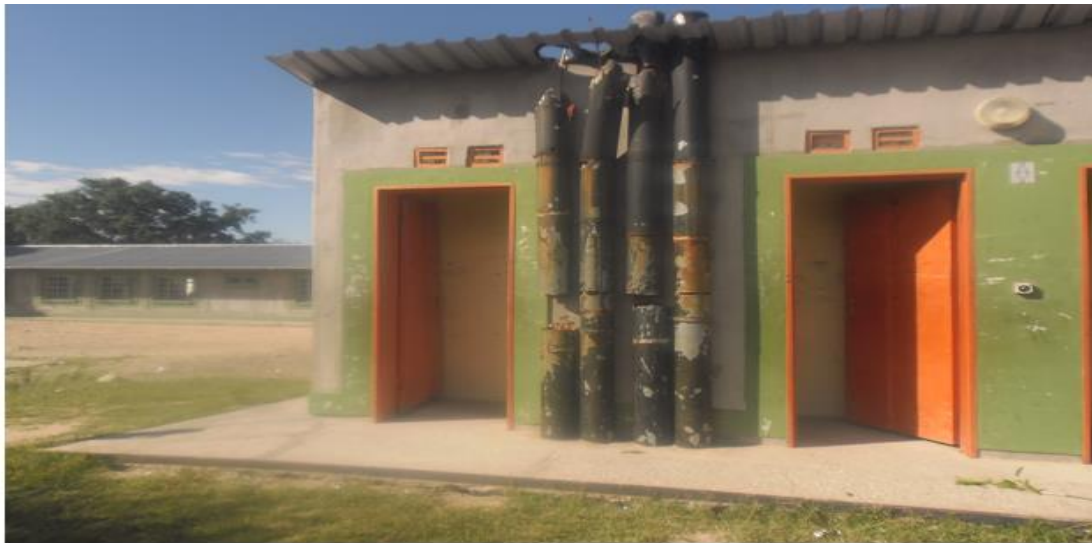
Figure 4.3: A toilet building with dilapidated vent pipes (source: researcher’s own picture).
