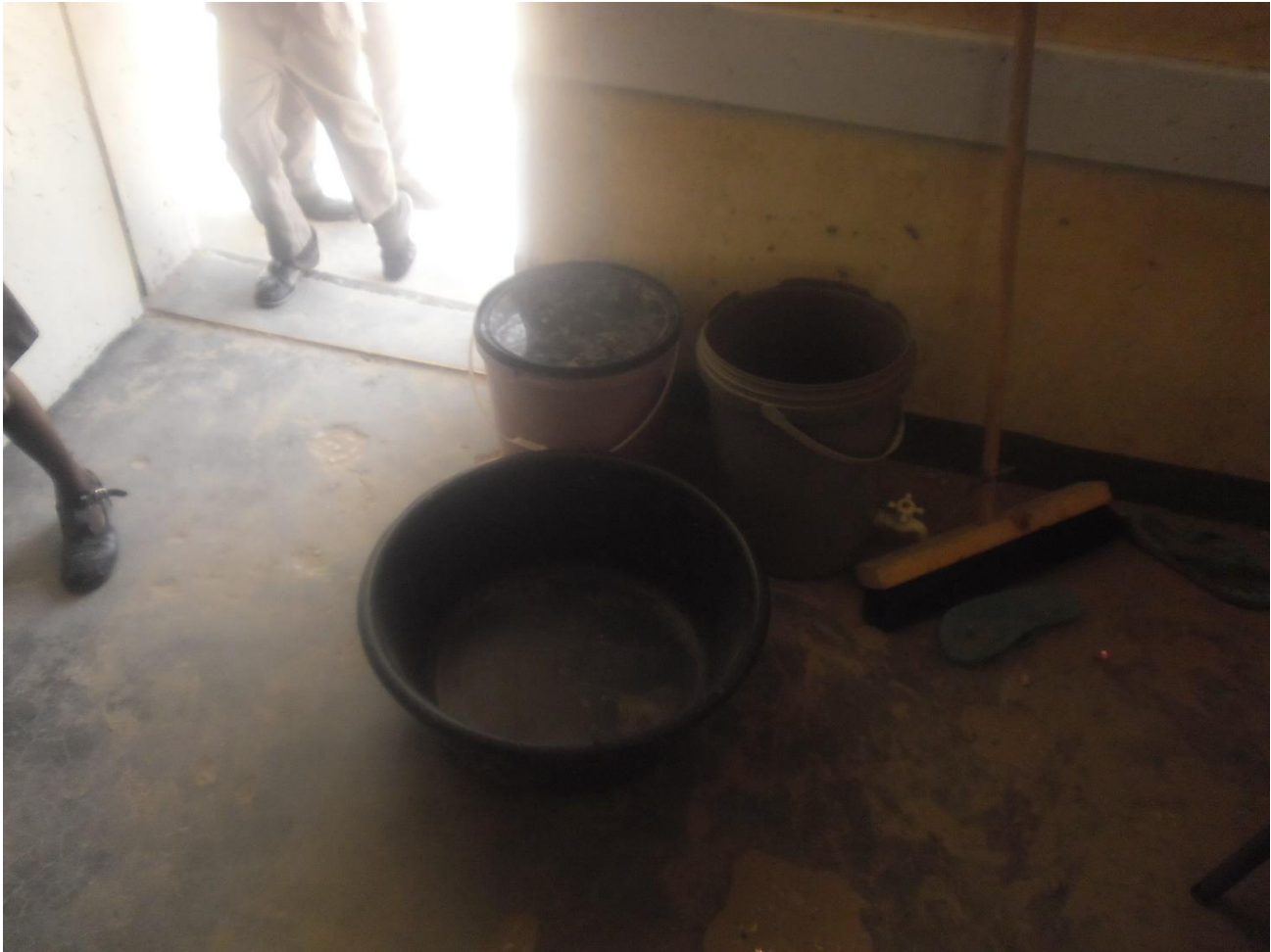
Figure 4.6: Unused handwashing facility (source: researcher's own picture).
