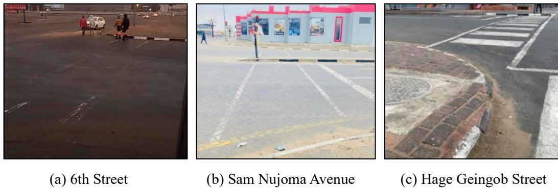
Figure 5.18: Absence of lowered kerbs at intersections
