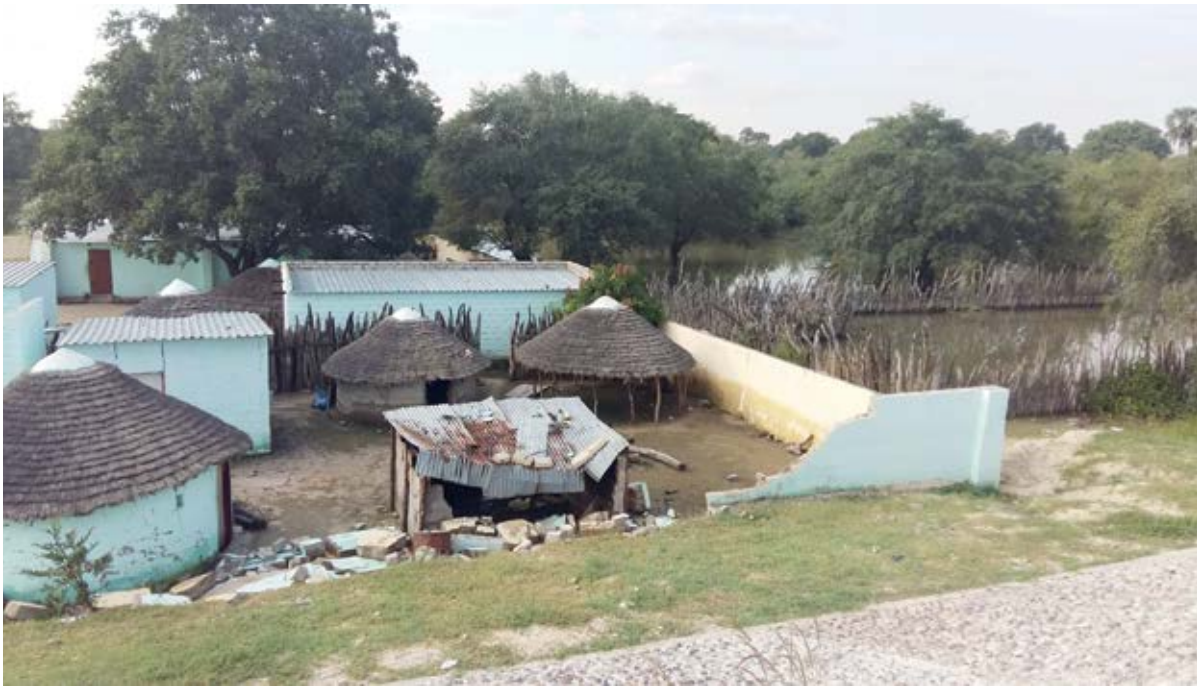
Figure 27: An example of a homestead damaged by flooding induced by the newly developed road near-by the homestead in the Cuvelai Basin. Note the water marks on the inner wall of the homestead.
