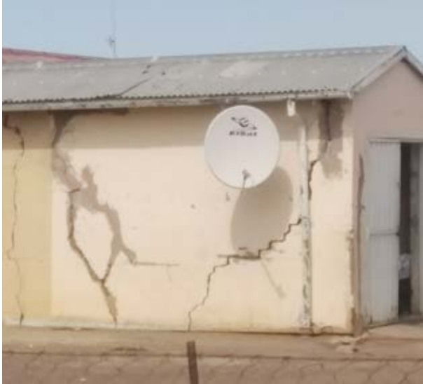
Figure 112: A house in Mariental with wall cracks, a phenomenon common in the town and affecting the property market in the area
