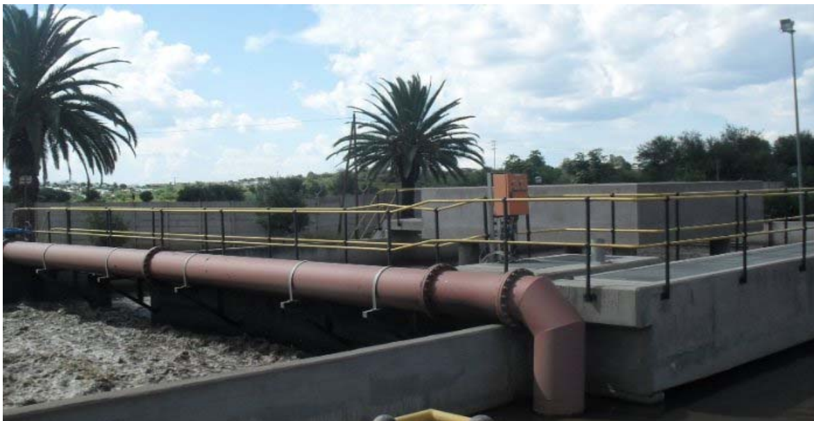
Picture 4: Part of the Gammams water care works.
