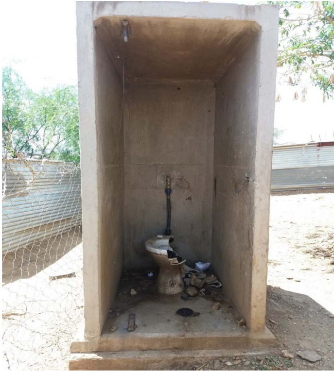
Picture 10: Broken Communal toilet with faeces on the floor in Havana Informal Settlement
