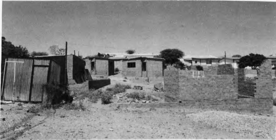
Photo 1: Incomplete houses: Khomasdal area
