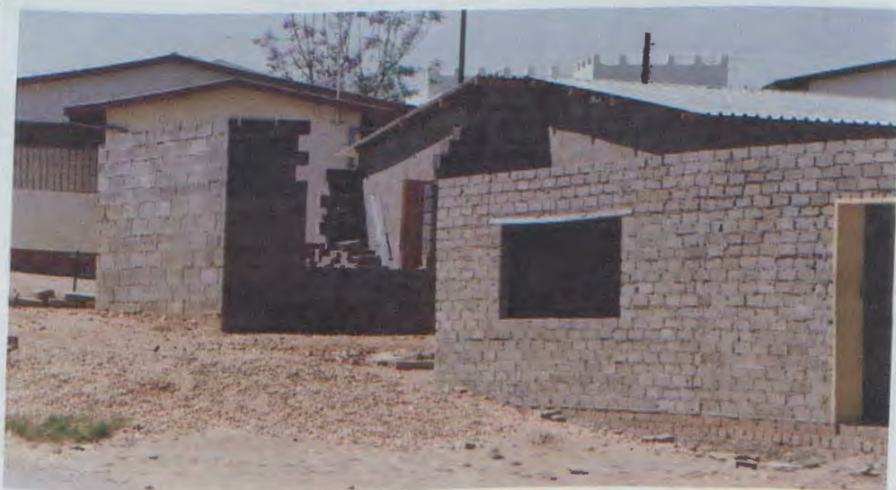
Photo 4: Incomplete houses of the Eagle group members: Khomasdal area
