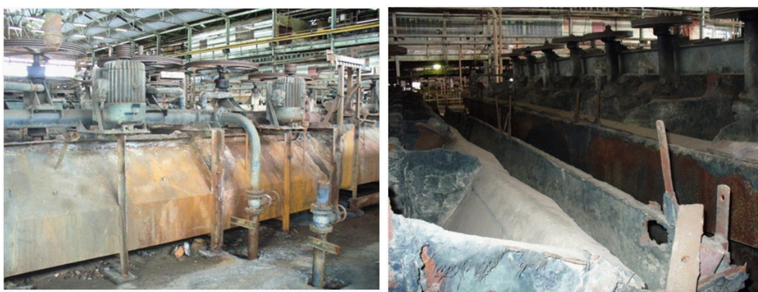
Figure 5.8: Two views of a dilapidated Gécamines flotation plant in Lubumbashi due to lack of reinvestment.
